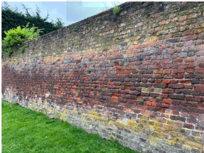
Historic brick boundary wall deteriorating from inappropriate use of cement mortars.
