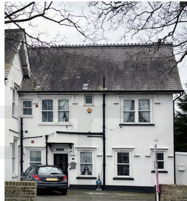
Modern uPVC rainwater goods detract from the aesthetic interest of this principal elevation.
