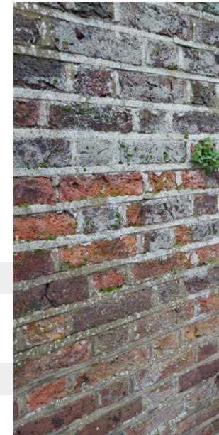
An example of ribbon pointing, efflorescence and vegetation growth affecting a brick wall
