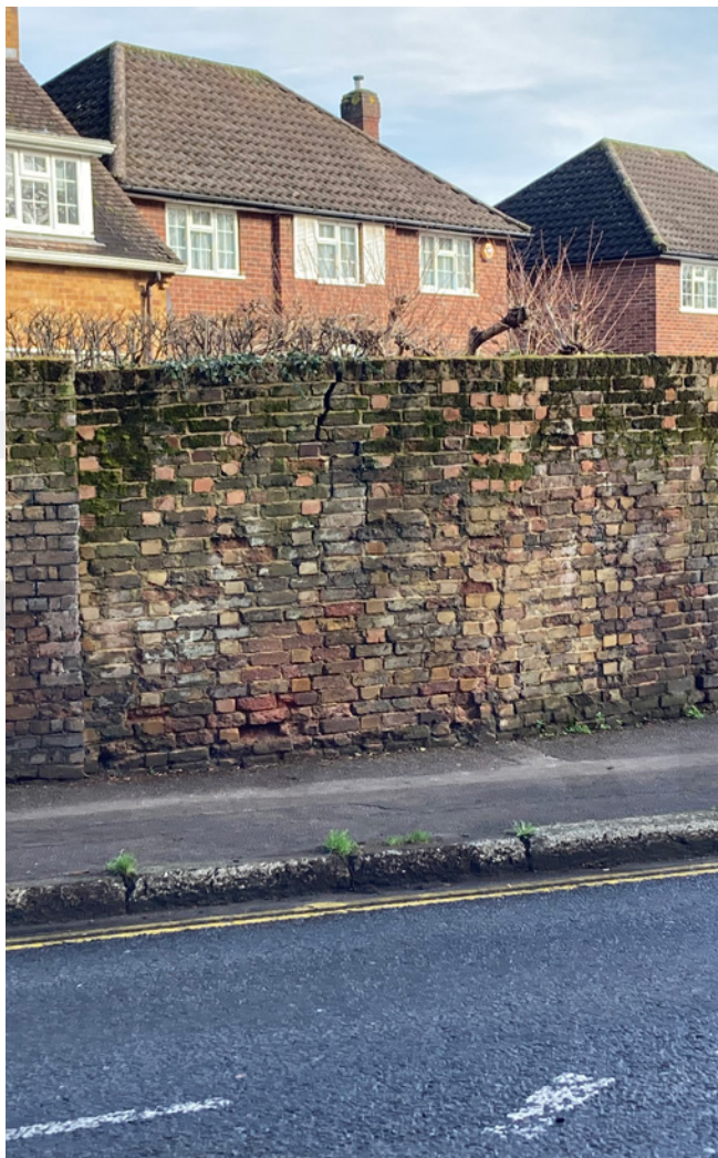
Many of the important brick boundary walls along the north side of Russell Road are in a deteriorating condition and in need of appropriate repair.
