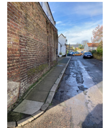
Example of the deteriorating surface condition to Ferry Square / Church Square.
