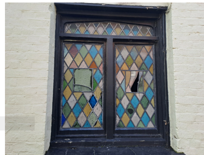
A characterful leaded light with stained glass to the Anchor Hotel, pictured from Church Road, in need of repair.
