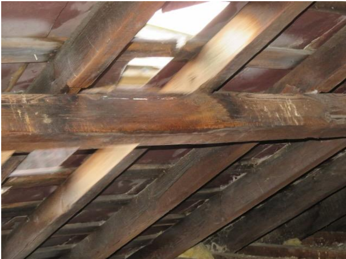
Photo 4- Holed Roof timber structure
