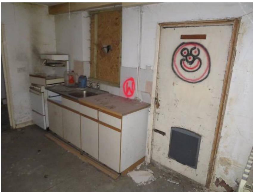
Photo 13- Guano covered derelict kitchen
