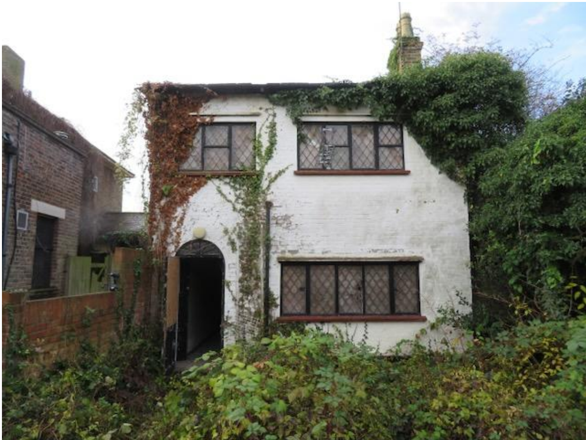
Photo 1- Front Elevation – Overgrown External walls
