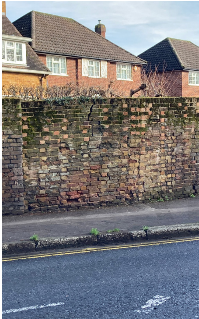
Many of the important brick boundary walls along the north side of Russell Road are in a deteriorating condition and in need of appropriate repair.
