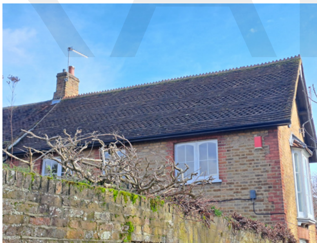
Decorative clay tiles to the roof of the Grade II listed Thamesfield Cottage on Russell Road.
