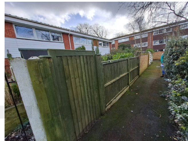
Inappropriate replacement of boundary treatments.
