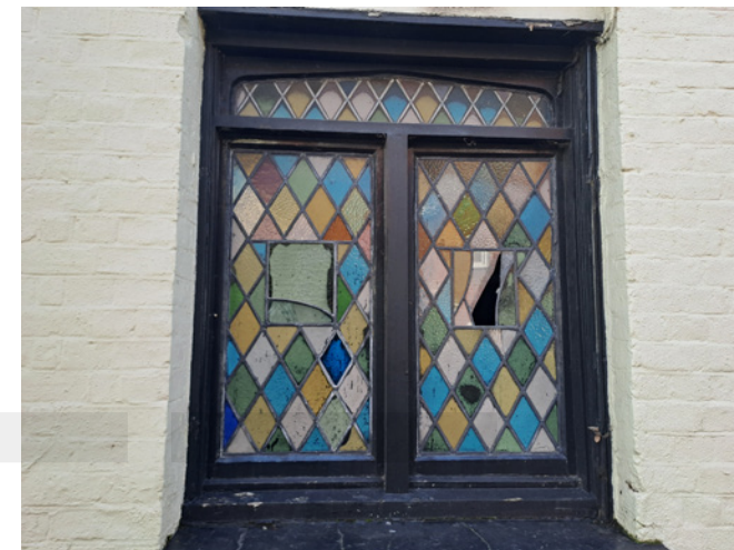
A characterful leaded light with stained glass to the Anchor Hotel, pictured from Church Road, in need of repair.
