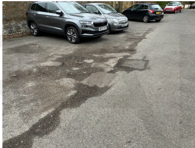
Potholed and uneven road surfaces detract from the visual appearance of the Conservation Area.
