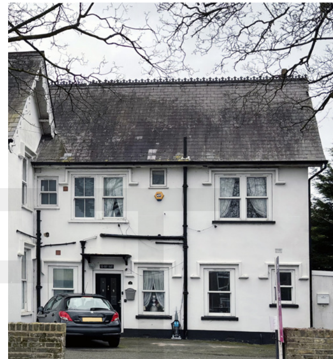
Modern uPVC rainwater goods detract from the aesthetic interest of this principal elevation.
