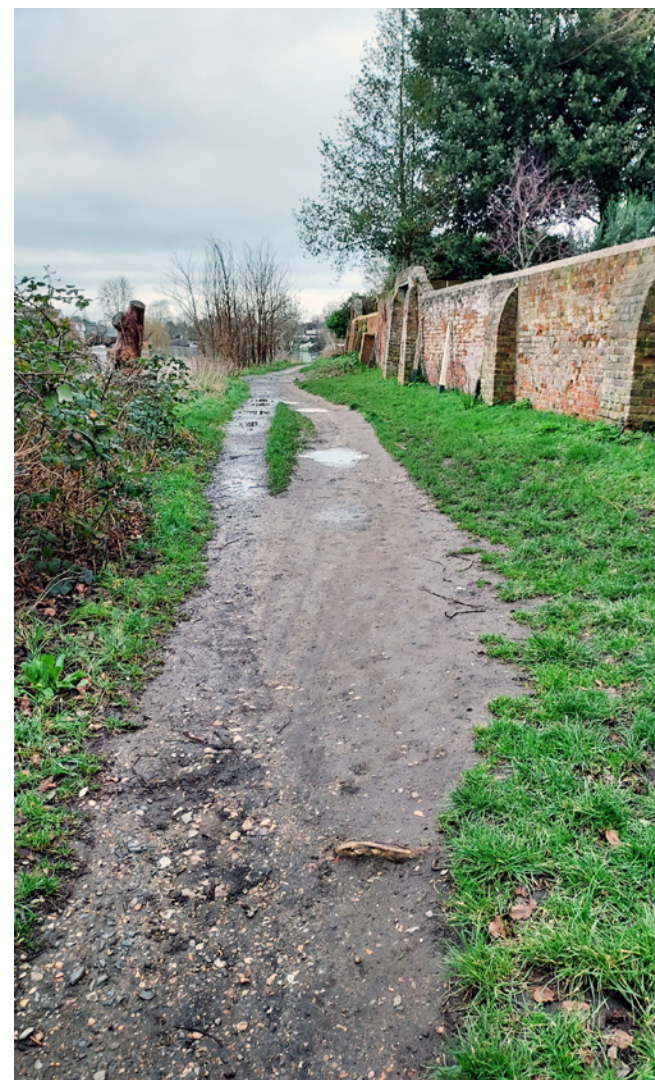
The listed brick wall along the northern portion of the Thames Side path
