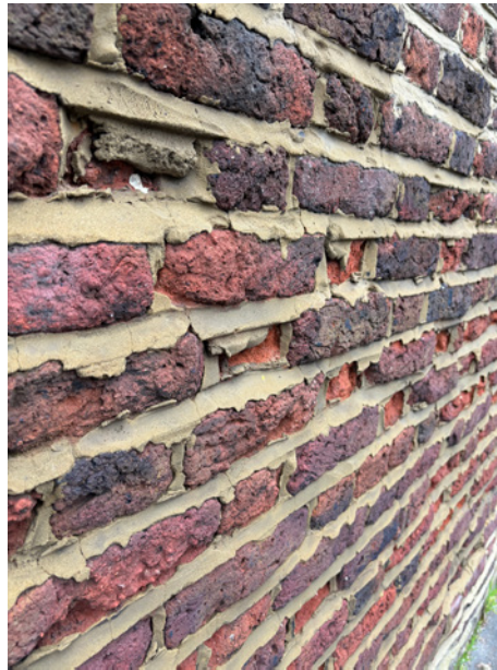
An example of ribbon pointing with cementitious mortar to a historic brick boundary wall in the Conservation Area.
