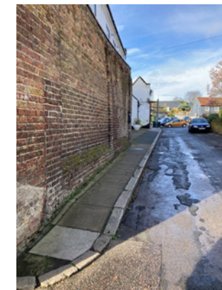
Example of the deteriorating surface condition to Ferry Square / Church Square.
