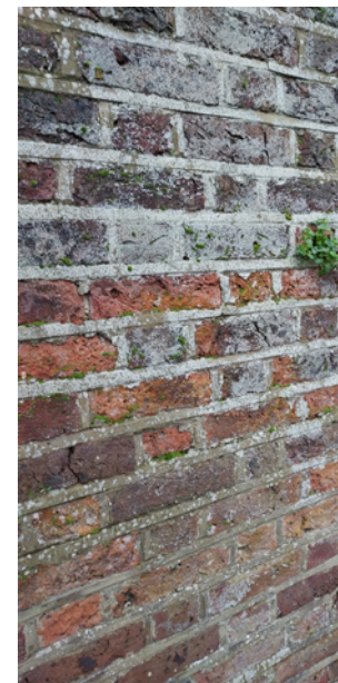
An example of ribbon pointing, efflorescence and vegetation growth affecting a brick wall
