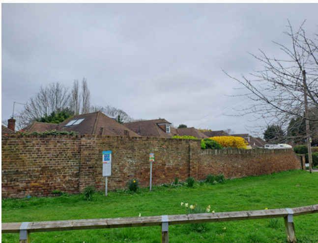
The brick wall separating nos. 1-8 Holmbank Drive from the village green, parts of which constitute the historic boundary wall of 42 Upper Halliford Road. The grounds of this large house were subdivided after 1934 to accommodate additional residential development along the northern side of the green.
