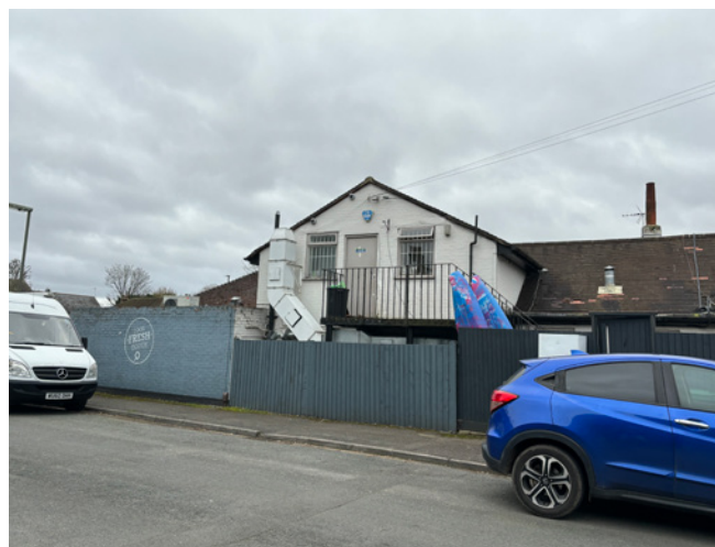
Visually prominent servicing and inappropriate timber fenced boundary treatment to the Goat Inn.
