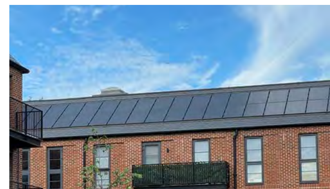
Flush photovoltaic panels incorporated into a roof
