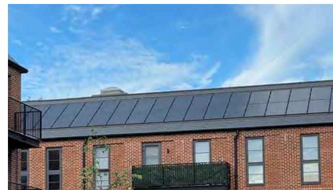
Flush photovoltaic panels incorporated into a roof
